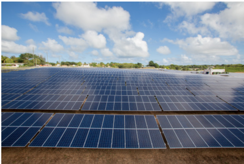
NRG Energy Spanish Town Estate Solar Facility, St. Croix USVI (Photo: Business Wire)
