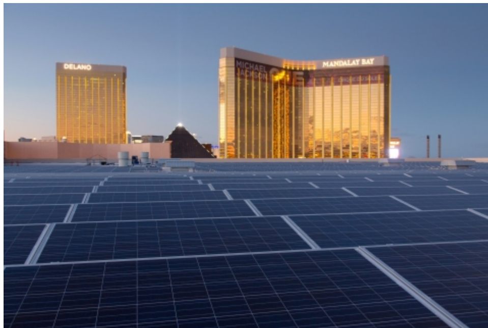
NRG Energy Solar Array at the Mandalay Bay Convention Center
